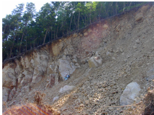
Fig. 2 Fractures within the weathered andesite at the Minamata landslide site (26 July 2003).
