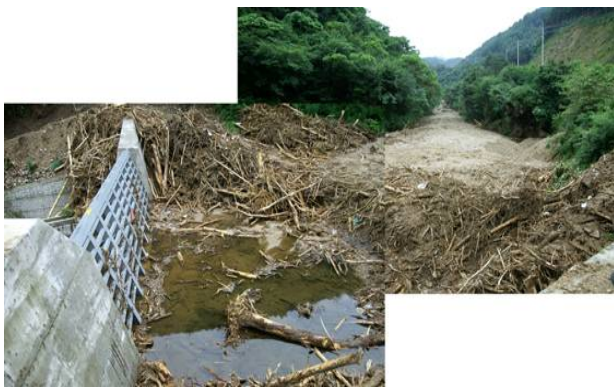
Fig. 12 Trapping debris flow and woody debris by construction of a buttress dam.
