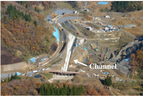
Photo 3 Landslide dam in Higashi-Takesawa area Photographed on 2005.11.21
