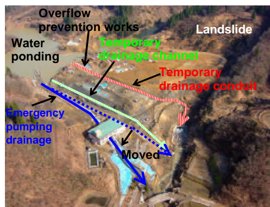
Photo 2 Emergency actions for the landslide dam in the Higashi-Takesawa dist. (Photographed on Dec. 14, 2004)
