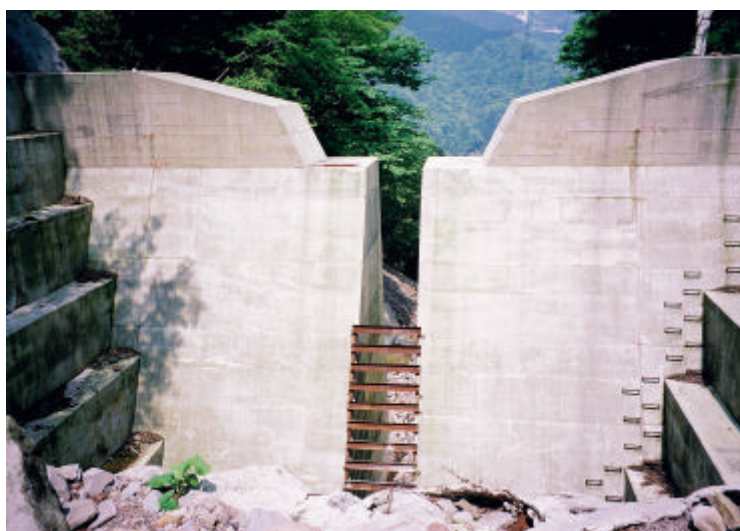
Photo 5 Concrete slit SABO dam. Steel bars were installed at the slit after debris flow passed through the slit.
