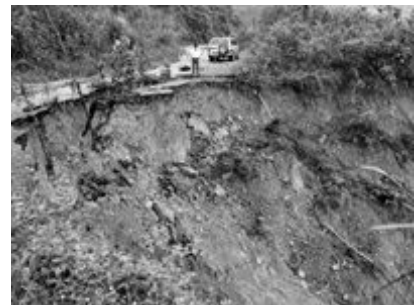
Fig. 1 Landslide occurred in Sa Pa district (above) and Bac Tra My District (below) in September 2013. Photo from http://www.news24.com/ and http://vietnamnews.vn/
