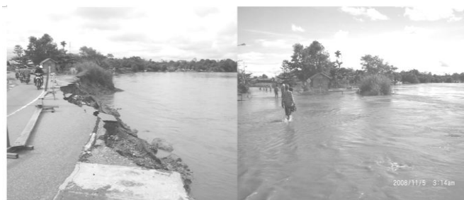
Fig. 3. Bank failure and flooding at Seluwing area
